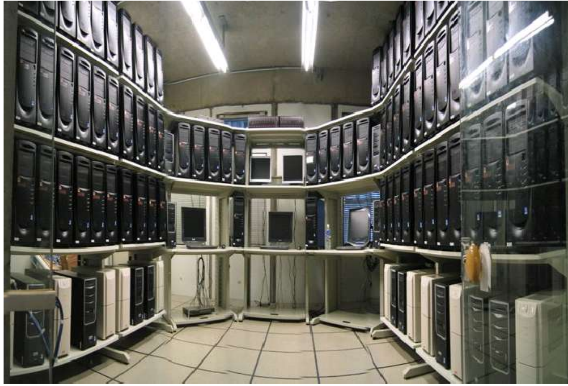
Figure 1 – The T2 HEPGRID BRASIL room at UERJ
